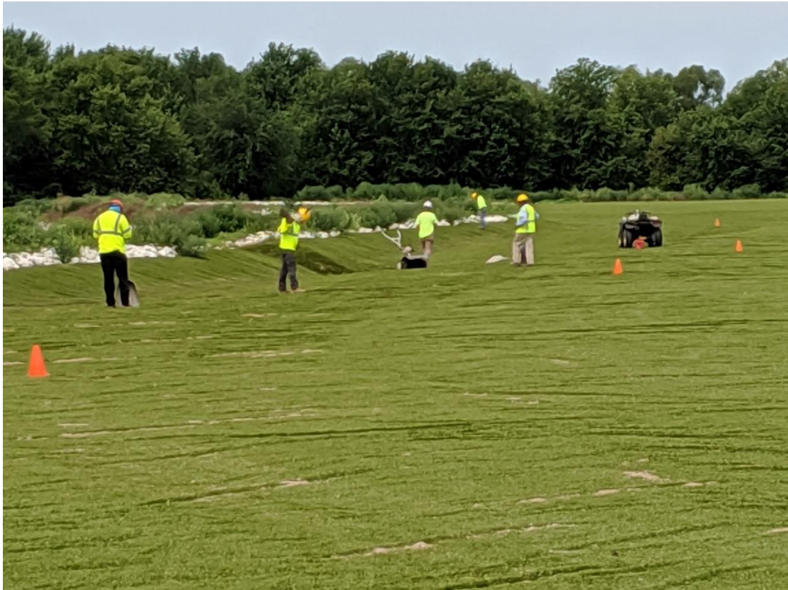
Photograph 2 ▲ - View of sand spreading activities in the perimeter ditch of the Fly Ash Pond, facing southwest.
